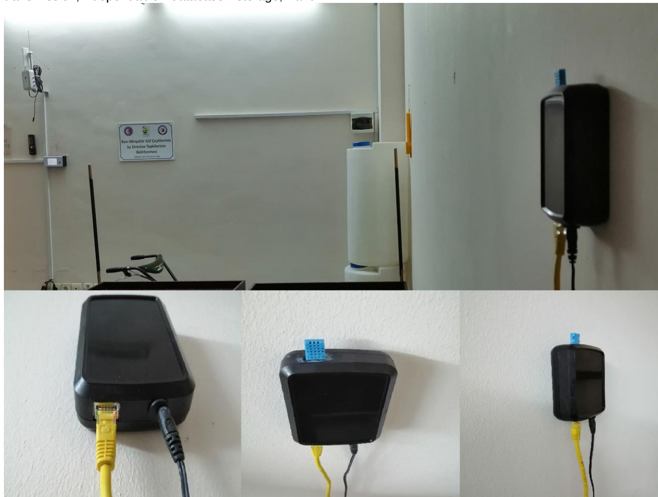
Figure 4. Installed device in detail.
